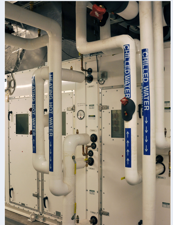
The Lakeview geothermal system, funded with help from USDA Rural Development, generates savings of about $350,000 in fuel costs annually.
